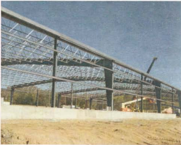
During the summer of 2007, Spec Building #3 in its early phases of construction.
