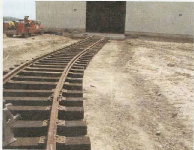
Rail construction also took place in The Point in 2007 adding to the already existing 7+ miles of rail.
