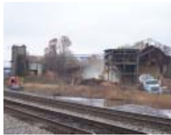
In late fall of 2006, crews tore down the old Carlyle Tile plant along US Route 52 in Coal Grove. The site is slated for use in an upcoming industrial development by McGinnis, Inc.
